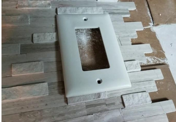
Pic 6: Switch plates on uneven texture walls
